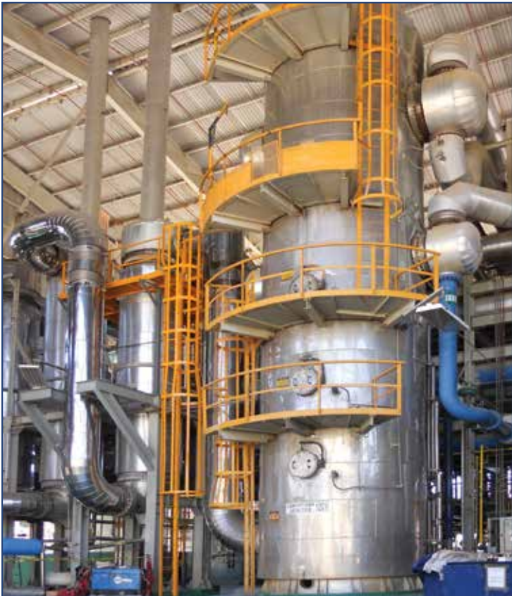
SO 2 -SO 3 Converter and SO 3 coolers
