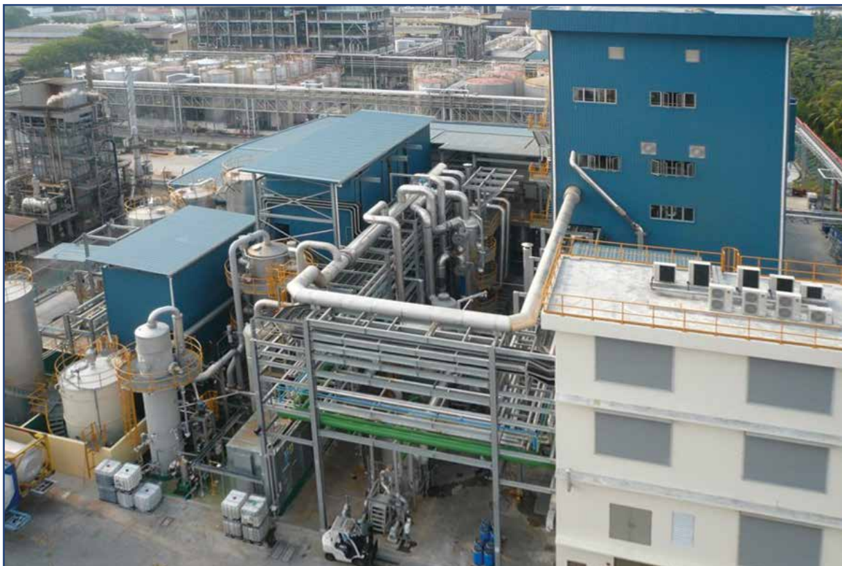
Sulphonation Plant Panoramic Views
