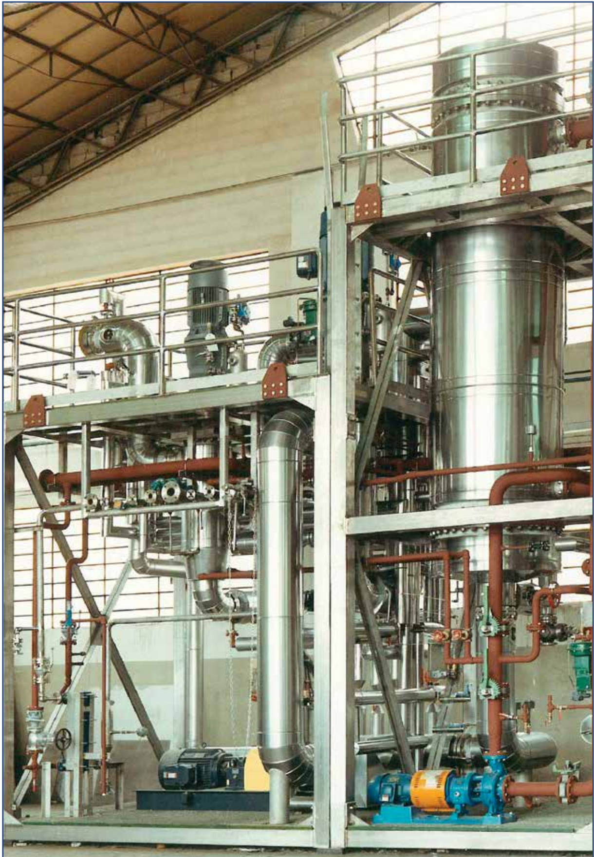
Skid-mounted Double Step Neutralization unit
